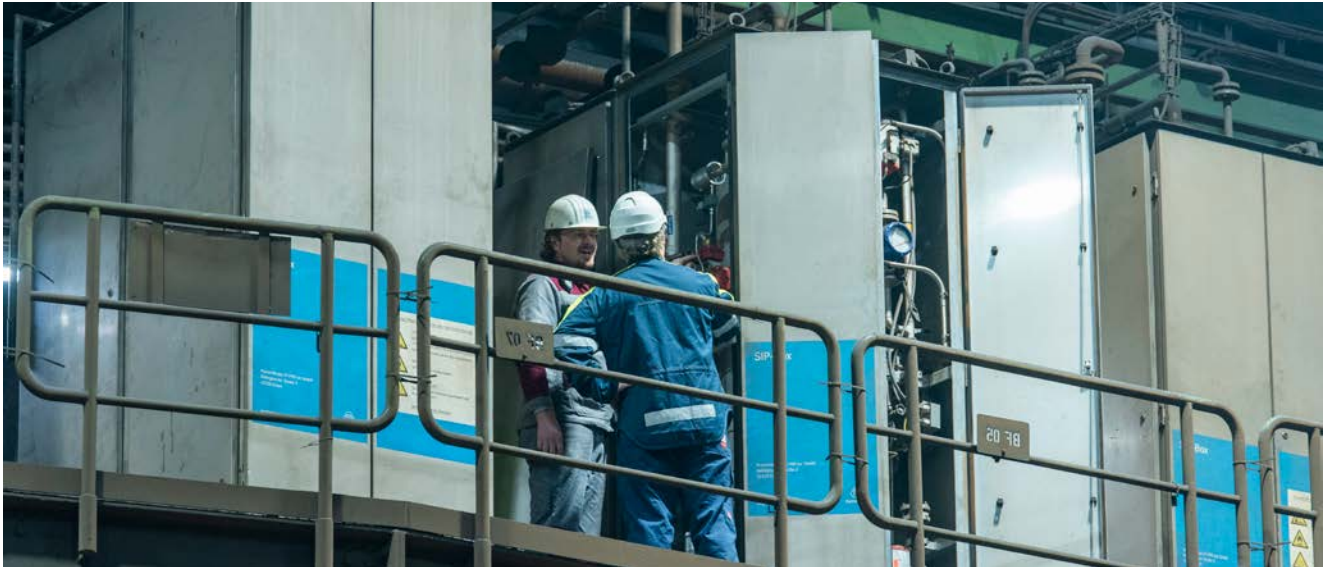
The SIP boxes are the result of many years of research and development: from the first tests at the Institute of Ferrous Metallurgy at RWTH Aachen, to the construction and optimisation of a prototype on the blast furnace in Schwelgern, to the installation of the complete SIP system during running operation.
