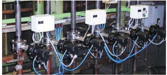
Sliding gate valves controlling the flow in an aluminium rolling plant: the aggressive and abrasive rolling emulsion is no problem for these valves which provide ultimate functional reliability by their two slotted plates sealing against each other. High-level leak-tightness despite suspended particles and a long service life create optimal conditions for economical production.
