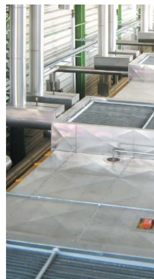
Drying plant in the Eberswalde pelletising plant for recyclable wood materials
