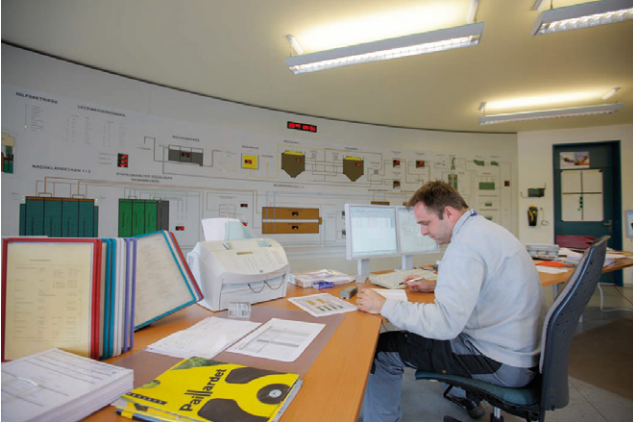
Control room at the Ros Sewage Treatment Plant, Wetzikon
